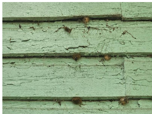
Exterior(008) B-Wall, Right Wood Wall Lead-Positive, Deteriorated
