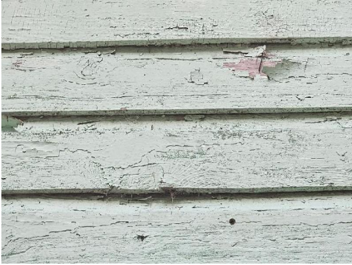
Exterior(008) D-Wall, Center Wood Wall Lead-Positive, Deteriorated
