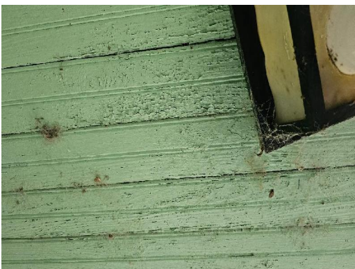
Exterior(008) B-Wall, Right Wood Porch Ceiling Lead-Positive, Deteriorated
